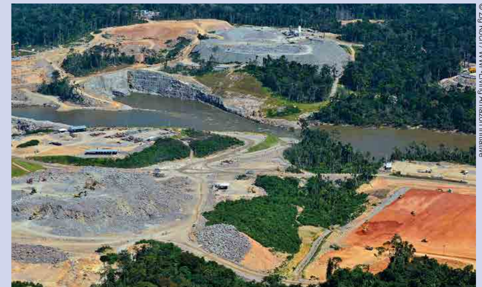
Teles Pires River being affected by dam construction, Mato Grosso state, Brazil.
